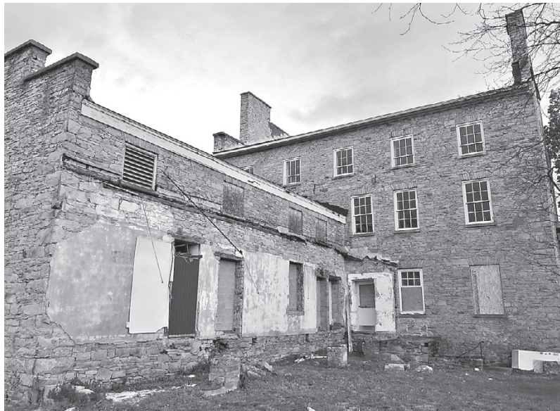
The back of 460 Center will have an elevator leading up to the top floors, as well as a rebuilt porch on the lawn.
