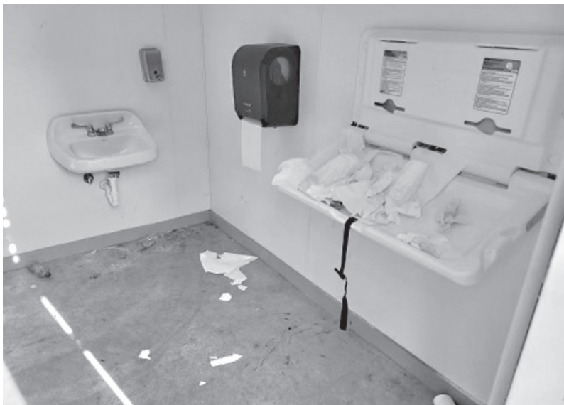
The playground bathroom was found in this condition. (Submitted) • New
