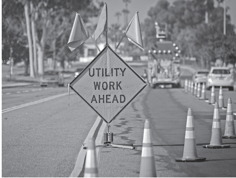
Image courtesy of National Grid
